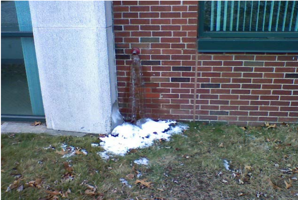
Photograph 3 - Unnamed Standpipe (23 January 2007)
