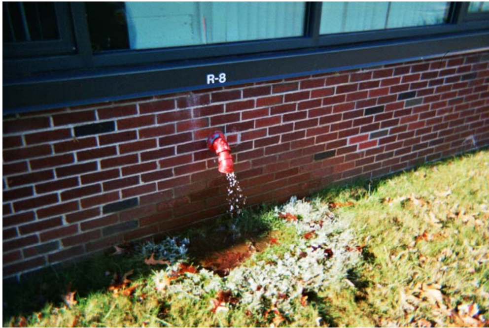
Photograph 1 - Leaking Standpipe R-8 (29 December 2006)
